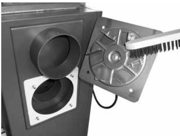
Sample cleaning of impeller and checking uprightness of vane on extract ventilator
